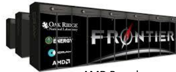
AMD Based (Up & running) 20 MW
