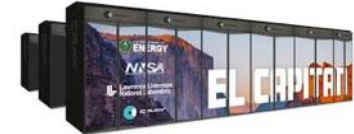
AMD APU Based (being commissioned)
